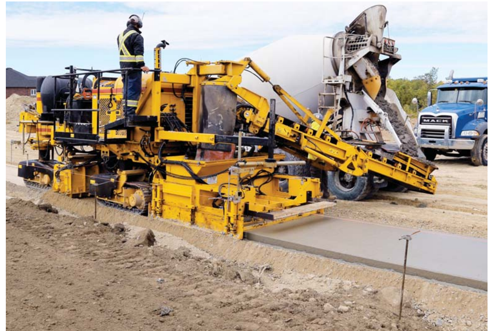
Curbside Construction says the GT-3200 sidewalk paver produces a high quality and precise sidewalk at a production rate far higher than what could be built by handforming.
